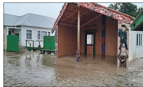
Tawhiti a Maru Marae was extensively damaged by floodwaters caused by Cyclone Gabrielle. Photo: Supplied
