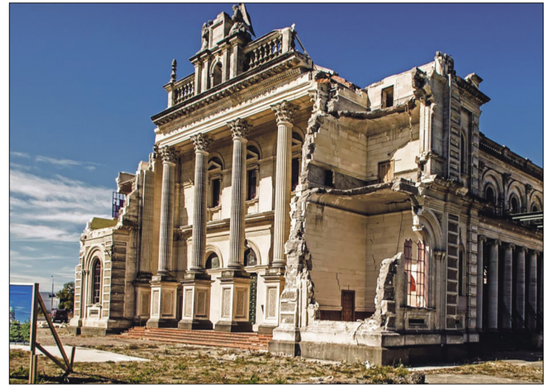
The ruined Cathedral of the Blessed Sacrament on Barbadoes St, before it was demolished in 2020. Photo: RNZ
